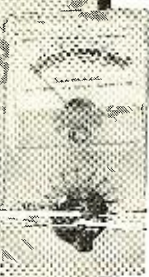
BATTERY CHARGE INDICATOR
